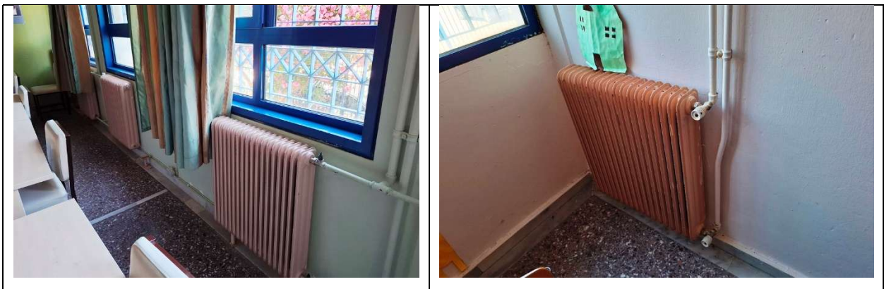
Figure 15: Existing steel radiators
